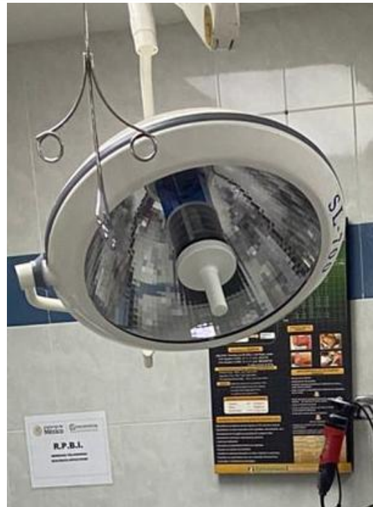
CEILING LIGHTS UPDATED AND NOT WORKING TIME AGO
